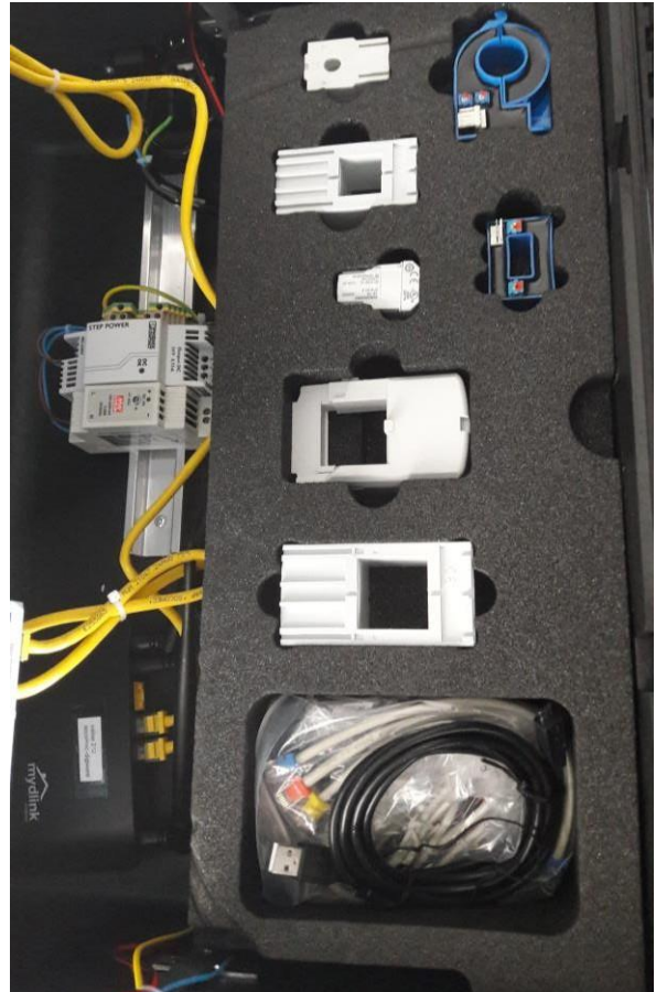
Inside : AC and DC sensors, Power supplies and router
